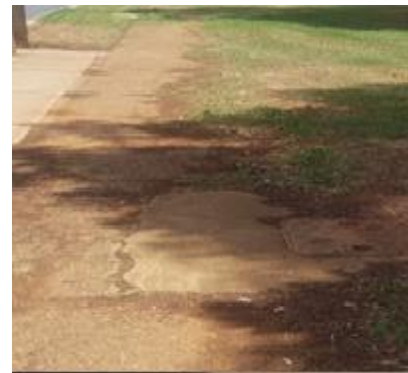
Figure 4.32: Pedestrian path, in bad state
